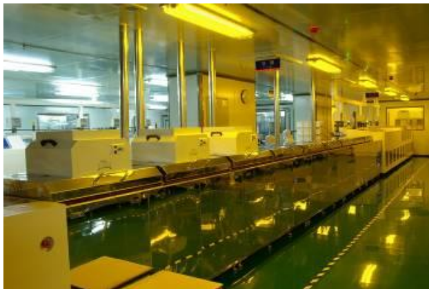
Developing and post baking line 1000 class clean room
